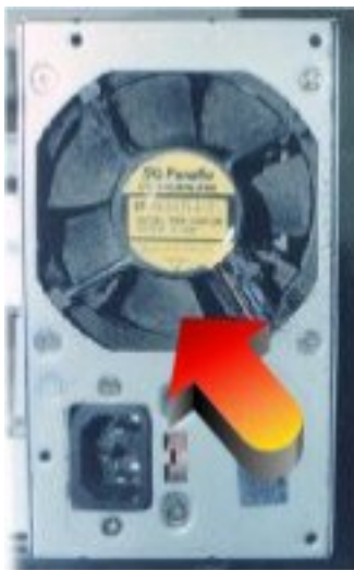
Close-up of PC cooling fan: note dust!
